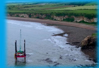
The project was delivered within the tidal zone from a 250 Tonne Jack Up barge.
