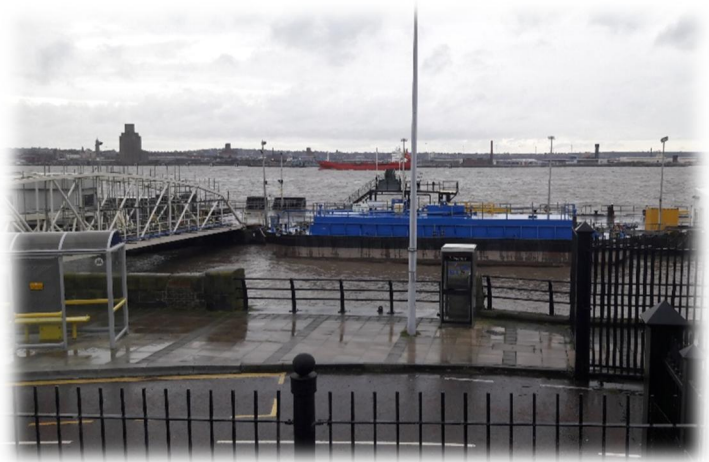
Steel and concrete repairs have increased the life span of the asset
