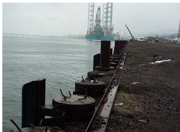
Upon completion of the former structure failure of a number of structural elements resulted in the works being deemed unusable.
