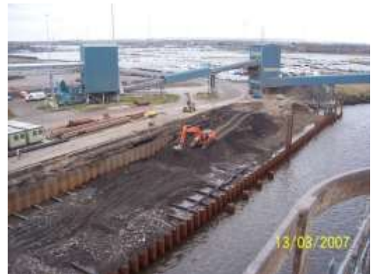
Sheet piled retaining wall with tie rods 300m length. Installation of rock armour & associated earthworks, 12,000m 3
