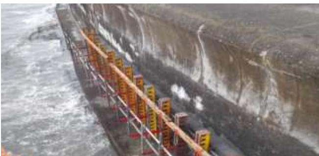
Skim wall construction. Access for Plant & Workforce via man basket. Material Access via Crane & Concrete Pump.
